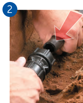
2 Ensure 2 threads are showing and simply slide the pipe in until the first point of resistance is felt.
